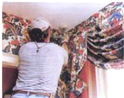
The system can supply central heating and cooling to historic properties without disturbing the historic details of the space.
