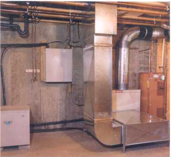
A 5-ton EarthLinked™ direct-access ground-source heat pump, from ECR Technologies, transfers energy from the earth, while a 5-ton Model ESP-V air-handling system, from SpacePak, heats and cools the home.
